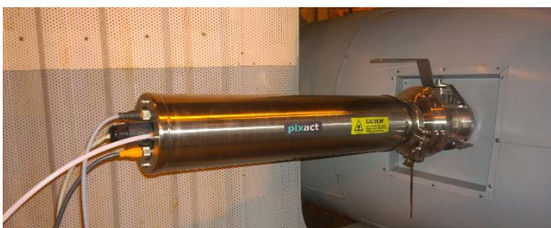
Figure 6. Pixact Bubble Monitoring system installed on the reactor inlet
